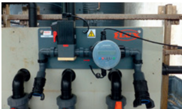
FMC 100 with switching amplifier FSV 100 installed in pipeline for semi-automatic filling.
